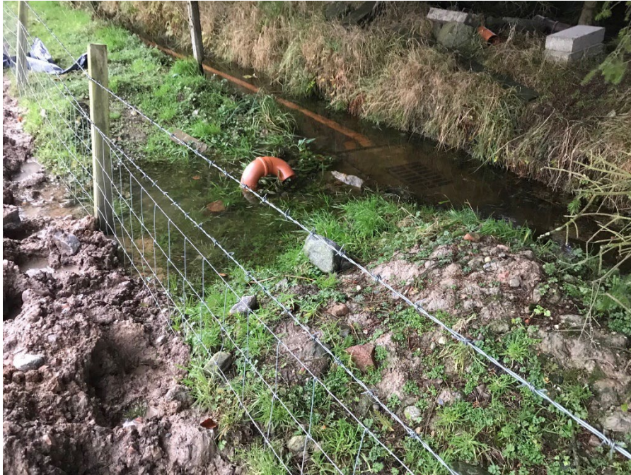
Figure 3 View of ponding at drainage outfall
